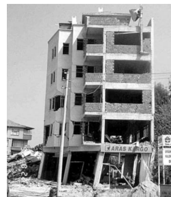
Fig. 1 Formulation of soft story mechanism during Turkey earthquake, 1999 (Sezen [8])
