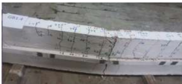
Figure (9): Shear failure of composite beam GB1.1
