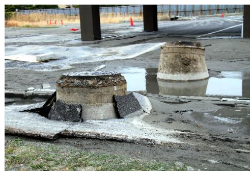
Figure 1 Manhole protruding by liquefaction
