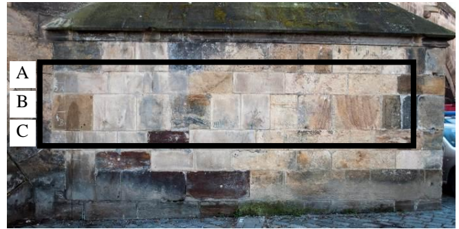
Figure 6. Trial assessment carried out in situ on three layers of sandstone masonry marked by the square.
