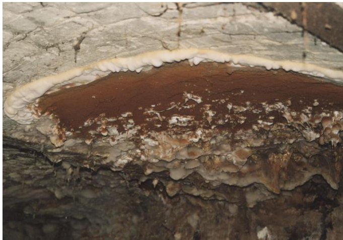
Fig. 5. The fruiting body of the house fungus proper ( Serpulla lacrymans ), grown into a vaulted ceiling of a basement room
