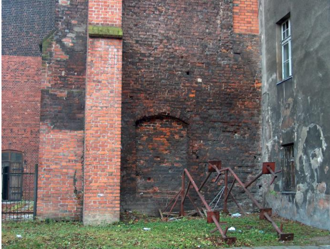
Fig. 3. Moisture level of the northern wall reaches approx. 5 m high above ground level - Museum in Raciborz.
