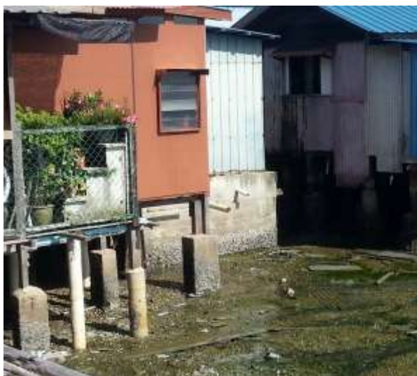
Figure 5 Human waste floating on the water surface
