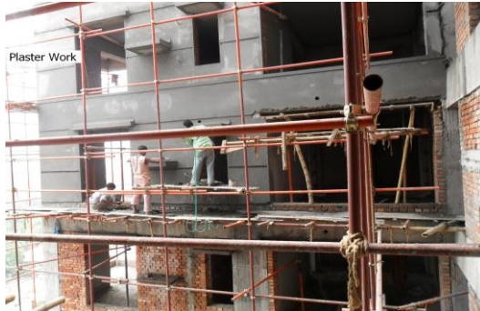
Figure 1. Workers working without any safety precaution (may cause fall accidents to the workers)
