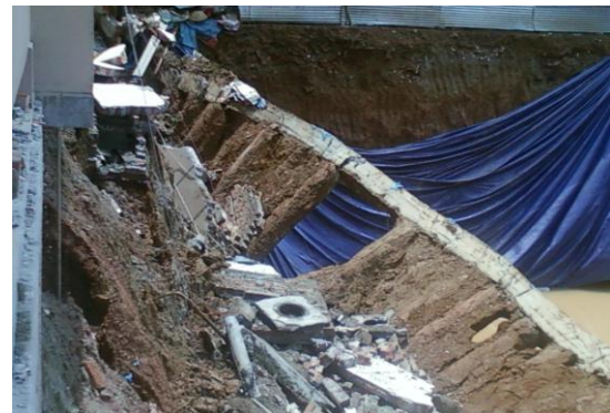
Figure 3. Trench collapse on a construction site
