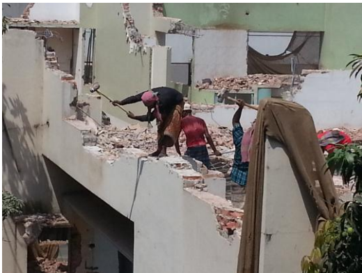
Figure 4. Unsafe condition during demolition work
