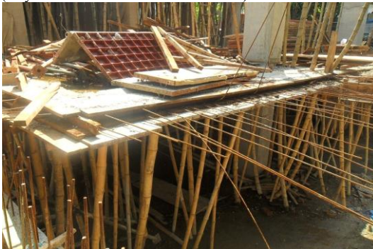
Figure 2. Bamboo props used as scaffolding and no safety net is present (may cause accidents to the pedestrians)
