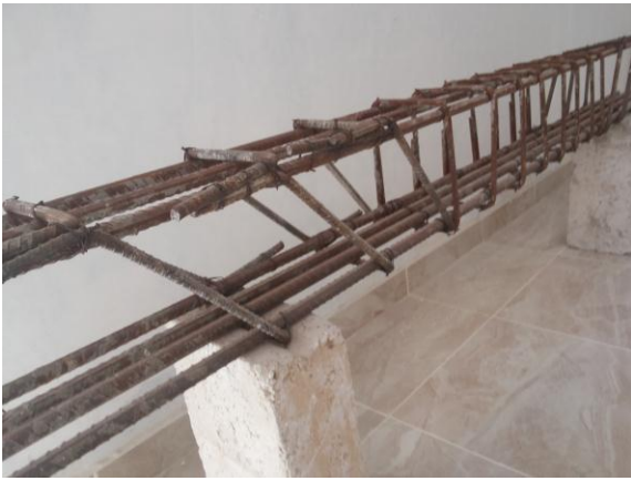
Fig. 3: Typical steel cage reinforcement of the beam reinforced with spliced swimmer bars.
