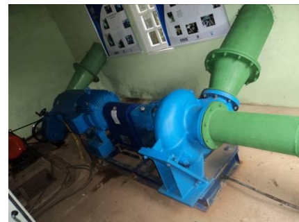
Figure 2: Pump as Turbine/Induction Generator group(Induction motor nameplate data: 45[kW], 60[Hz], 220/380/440[V], 1780[RPM], power factor: 87%, efficiency: 93.1%, manufacturer: WEG)
