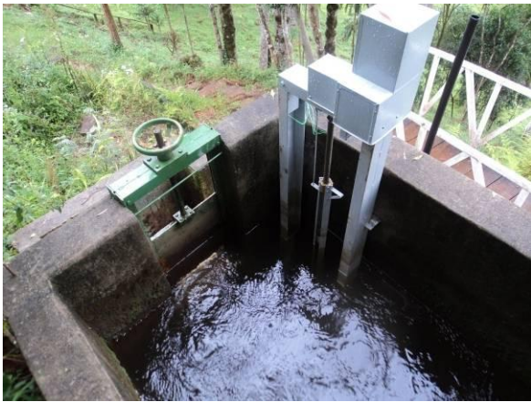
Figure 8: The floodgate at right is actuated by a DC 24[V] motor located at the top. This voltage is supplied by batteries. The entrance of the pipe is located under water.
