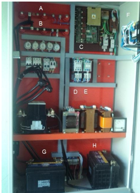
Figure 12: Power house cabinets (Legend: A - positive bar; B - negative bar; C - Semikron MP410T board; D - K1 contactor for floodgate descent; E - K2 contactor for floodgate rising; F – under-voltage and overvoltage relays; G and H - batteries).
