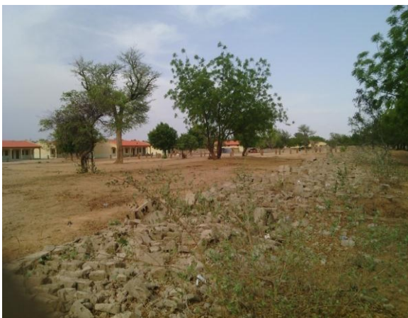
Plate 3: Collapsed block wall fence around public School
