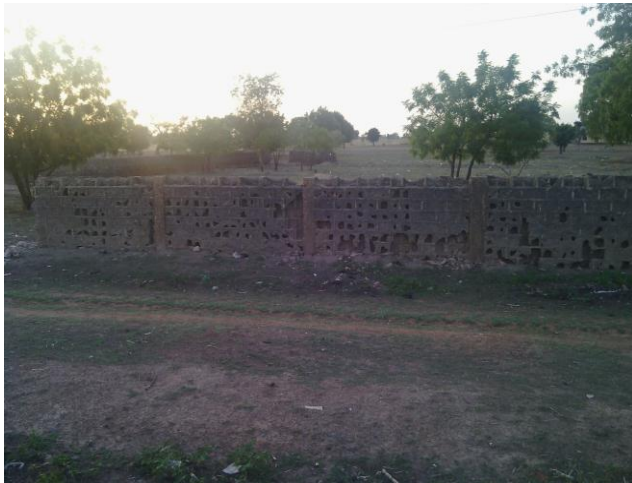
Plate 2: Wall built with poor Quality Blocks
