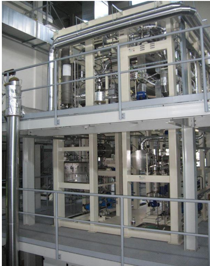
Figure 1. Supercritical water loop in Research Centre Rež. Active channel (vertical pipe in the very left is still in out-of-pile operation)
