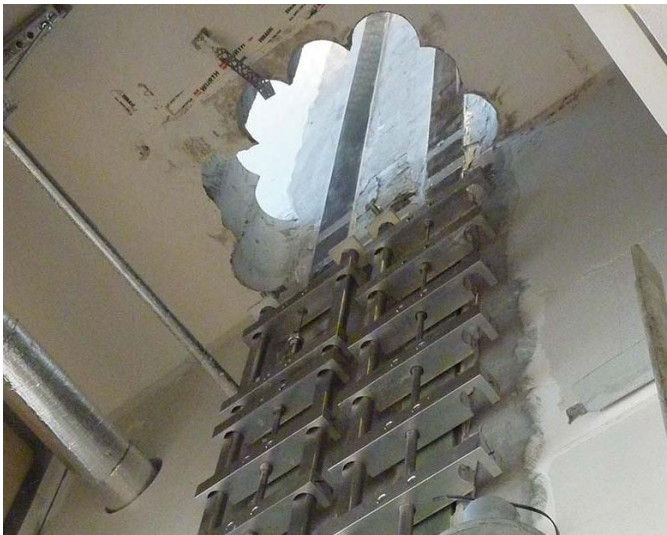
Figure 8. Strengthening of a wall in a hotel building in Sweden with four laminates, pre-stressing force of 65 kN in each laminate.
