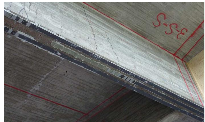
Figure 7. Strengthening of The Gruvvagen bridge in Sweden with three laminates, pre-stressing force of 110 kN in each laminate.
