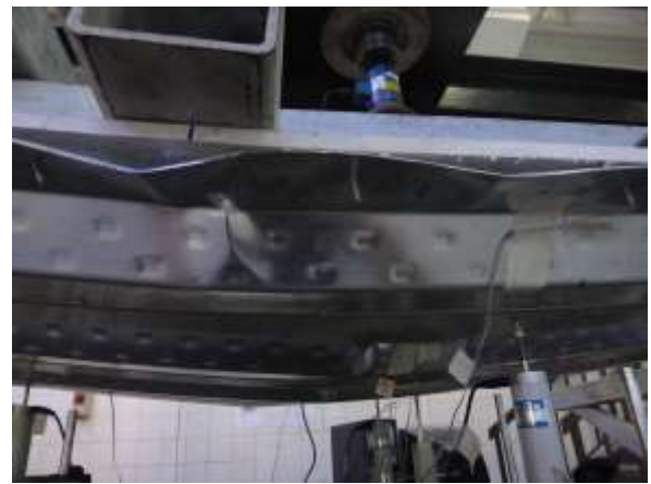
Figure 6 Local buckling for FBNC sample
