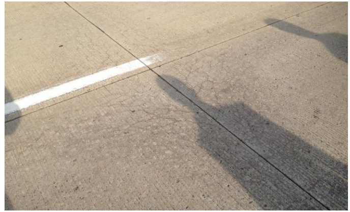
Figure 1. Map cracking in pavement.
