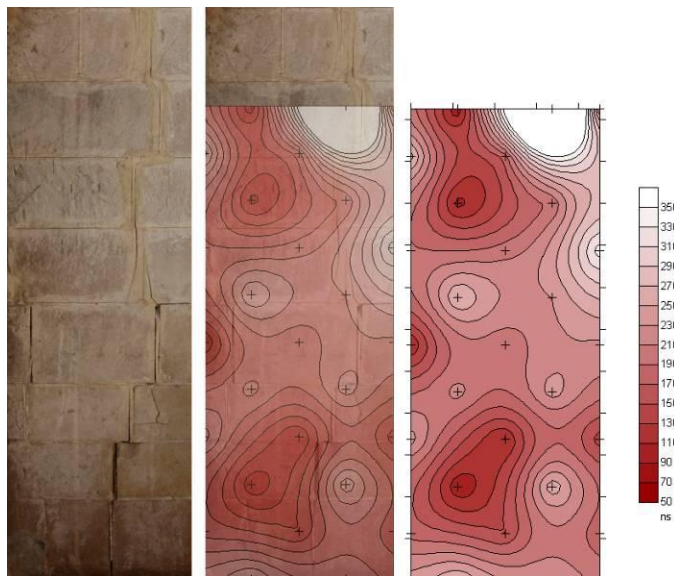
Figure 13. A lesion in the wall near the entrance central portal. Ultrasonic tomography processed with the measurements of pulse propagation time between the probes.
