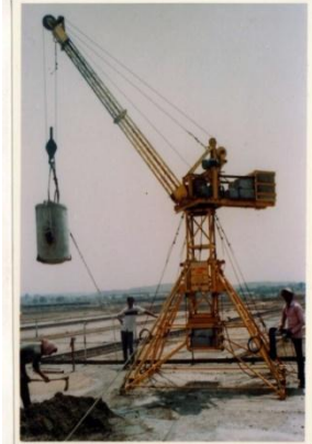
FIG.06 : HELPING BASE CONCRETING OF WALL FOUNDATION FOR COAL HANDLING PLANT AT SUPER THERMAL POWER STATION, CHANDARPUR (MS).
