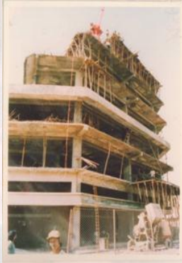
FIG.02 : EIGHT STOREYED POONAM TOWER UNDER CONSTRUCTION AT NAGPUR AND MINI CLIMBING CRANE HELPING IN LIFTING CONCRETE FROM THE MIXER PLACED ON THE GROUND.
