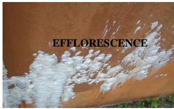
Figure 2: Efflorescence on concrete wall
